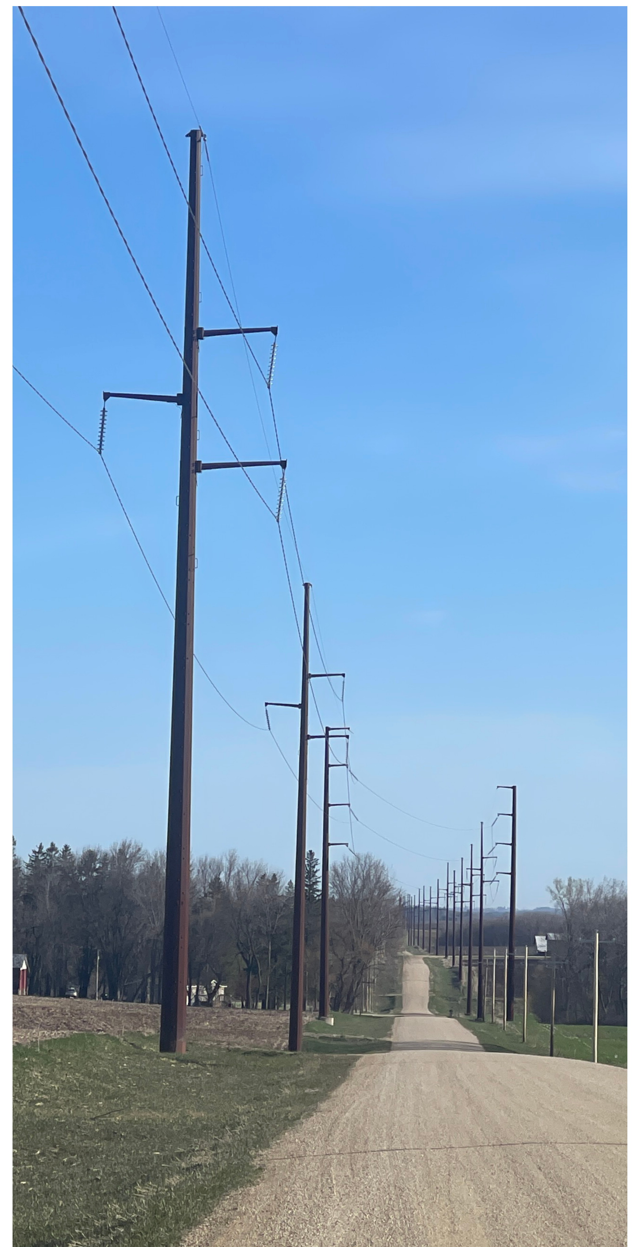
This picture includes an existing 161 kV transmission line.
